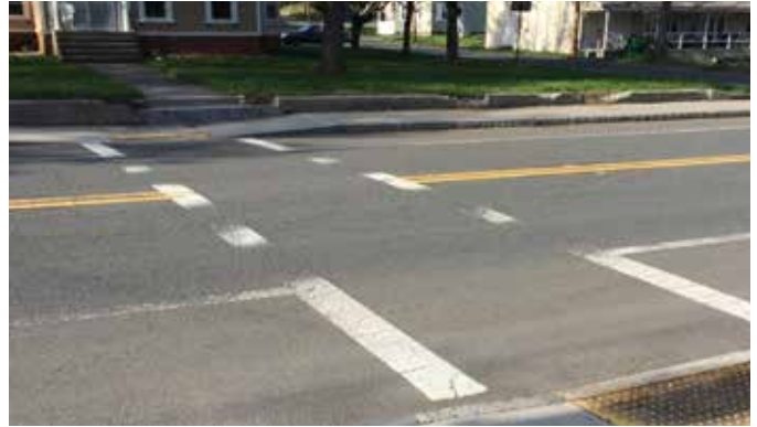
Crosswalks on Route 112 currently do not have in-street pedestrian signs to alert drivers to the possibility of people crossing
