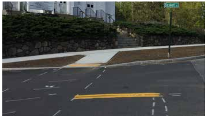
Ladder crosswalks are planned to complete the recent curb bump out construction at the Basket/Maple Street intersection with Route 112.
